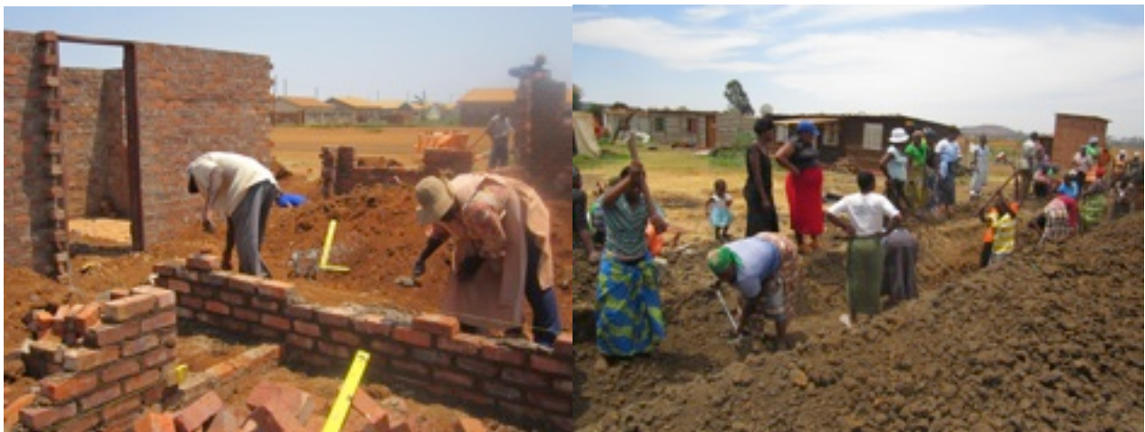
Women bricklayers working alongside their male counterparts while other Federation women work on the trenches for the open culverts for storm water drainage
