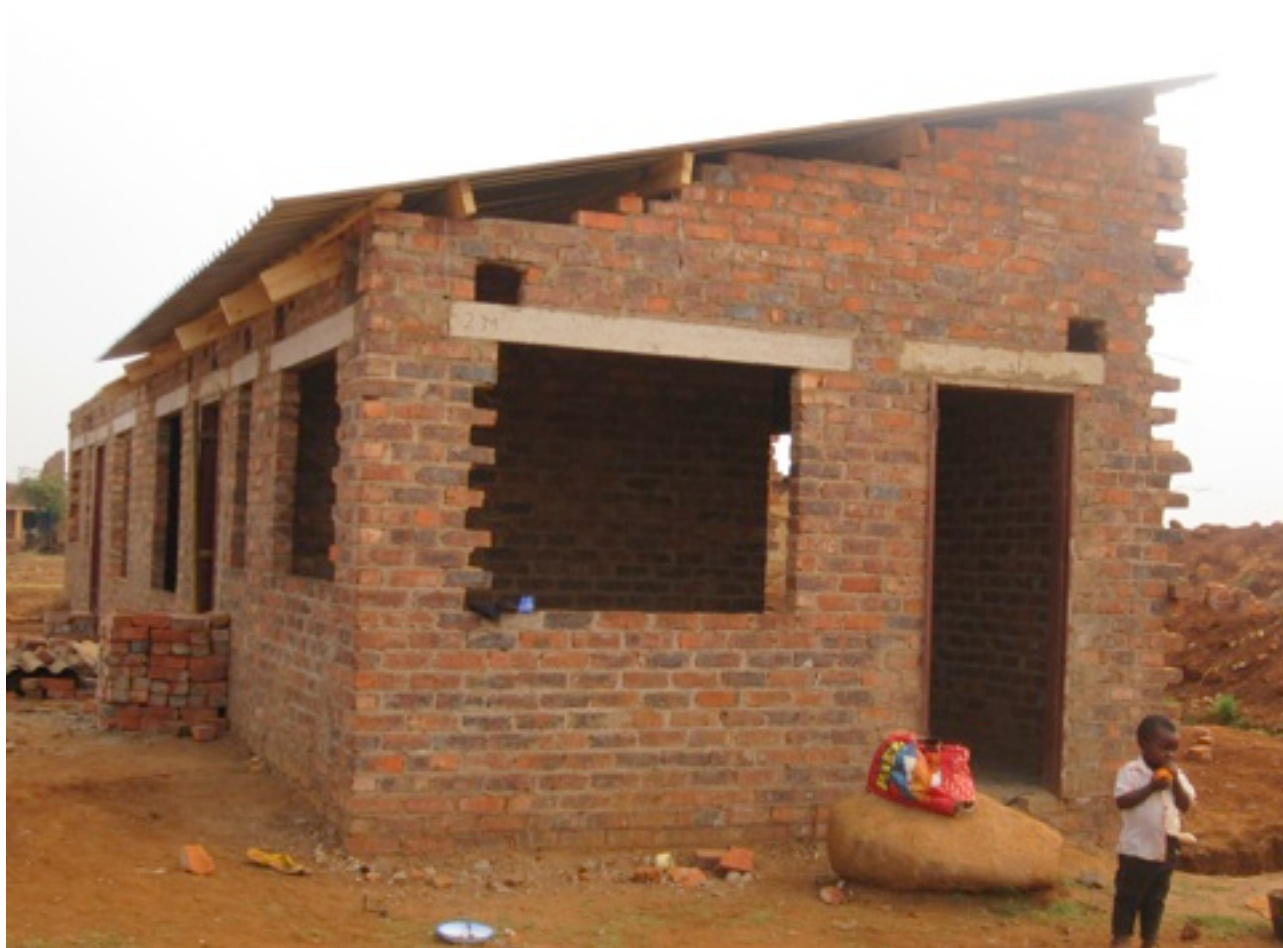
Picture depicting some of the densification house models currently at roof level in Dzivarasekwa Extension
